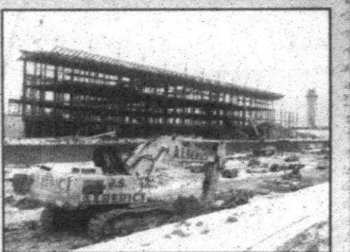
Concrete and steel: The new Midfield Terminal rises near Metro's control tower (far right) as road-building continues.
