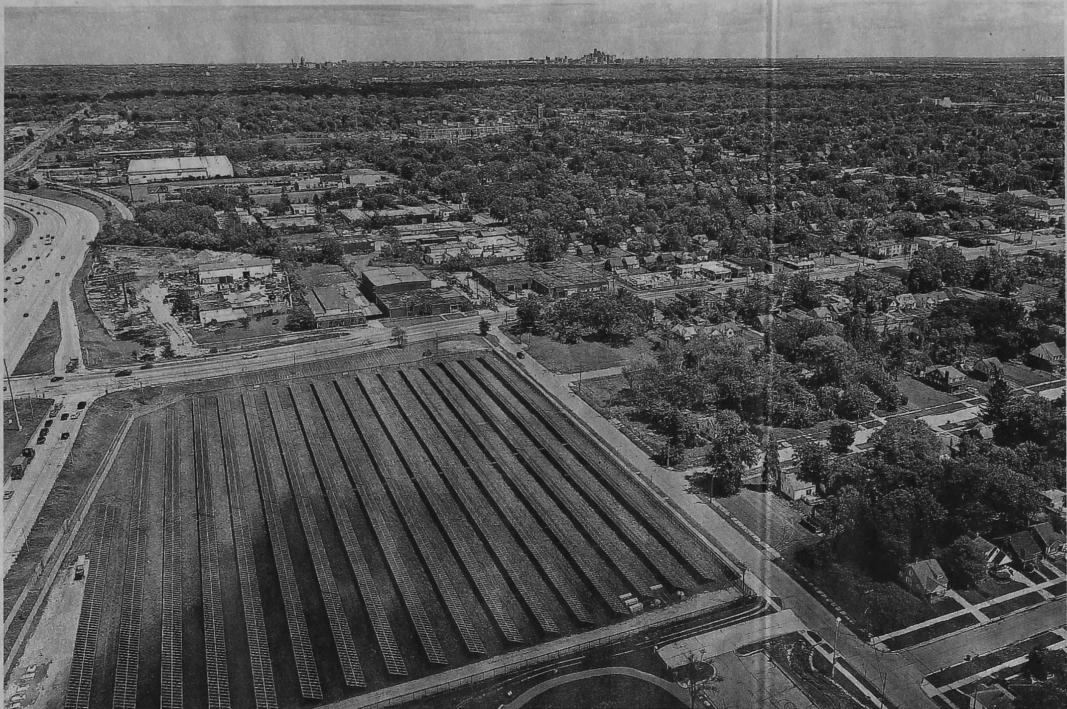
Solar panels at the DTE O'Shea Solar Park are located at Greenfield Road and Capitol Avenue in Detroit, just south of Interstate 96. The solar park's 7,400 panels produce enough electricity to power the equivalent of 450 homes with clean energy. KELLY JORDAN AND MANDI WRIGHT/DETROIT FREE PRESS
