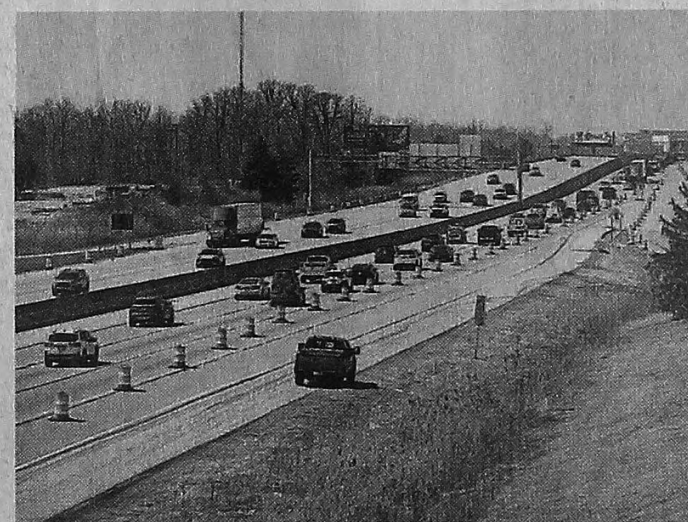
Westbound I-96 near Novi is part of a reconstruction effort by MDOT. HOMETOWNLIFE.COM FILE
