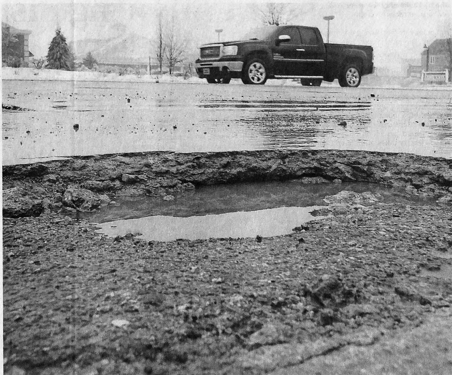
A pothole four inches deep with sharp rim lies along Canton Center Road's northbound lane. JOHN HEIDER/HOMETOWNLIFE.COM
