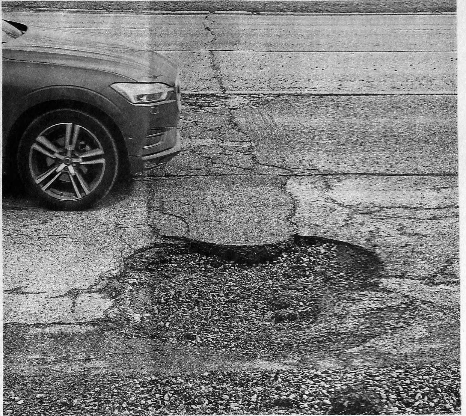
A substantial pothole in the southbound lane of Haggerty as it approaches Seven Mile. JOHN HEIDER/HOMETOWNLIFE.COM
