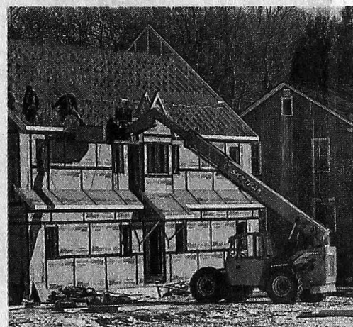
A market-rate housing development is under construction at 175 James St., a former brownfield.
