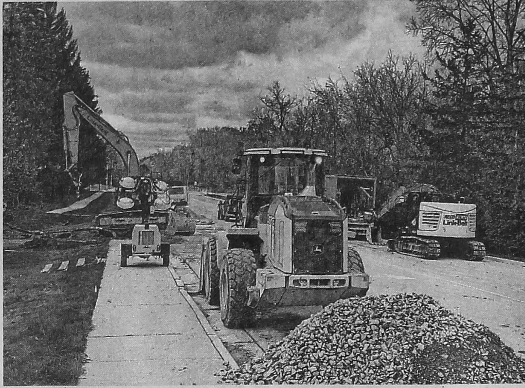
Crews work to repair a 48-inch water main break along 14 Mile Road on Monday.
