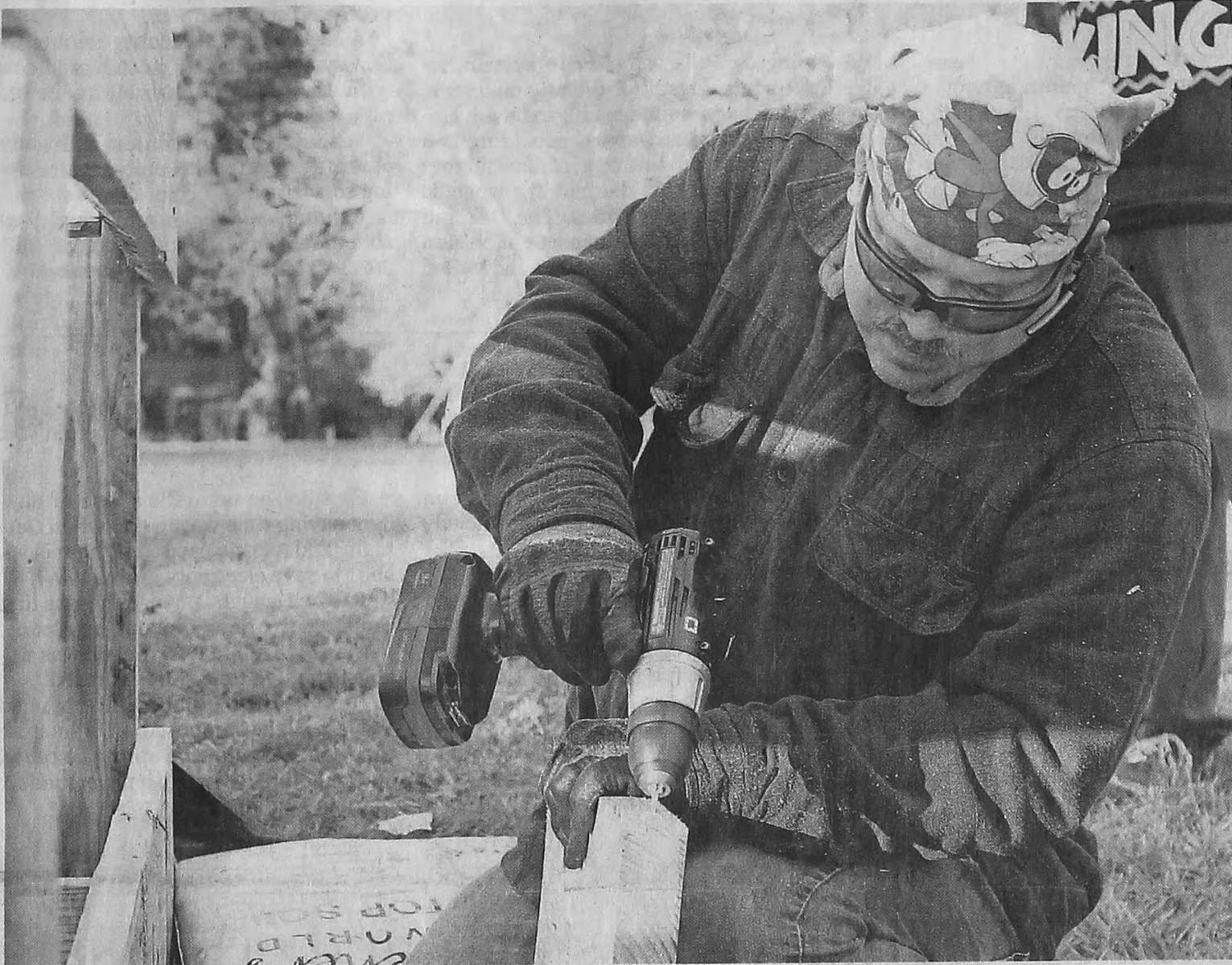
Faith Wesleyan Community Church Lead Pastor Tom Hazelwood works on building the church's new garden boxes. JOHN HEIDER/HOMETOWNLIFE.COM
