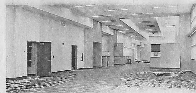
Inside the Veterans Affairs clinic under construction in Canton Township. COURTESY OF U.S. VETERANS AFFAIRS
