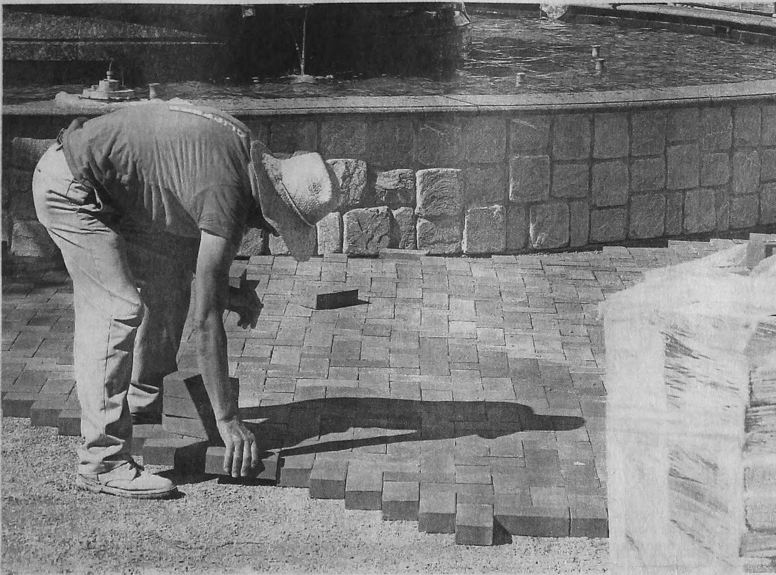
A worker installs a brick walkway at the Kellogg Park fountain Sept. 27 in Plymouth. PHOTOS BY JOHN HEIDER/HOMETOWNLIFE.COM
