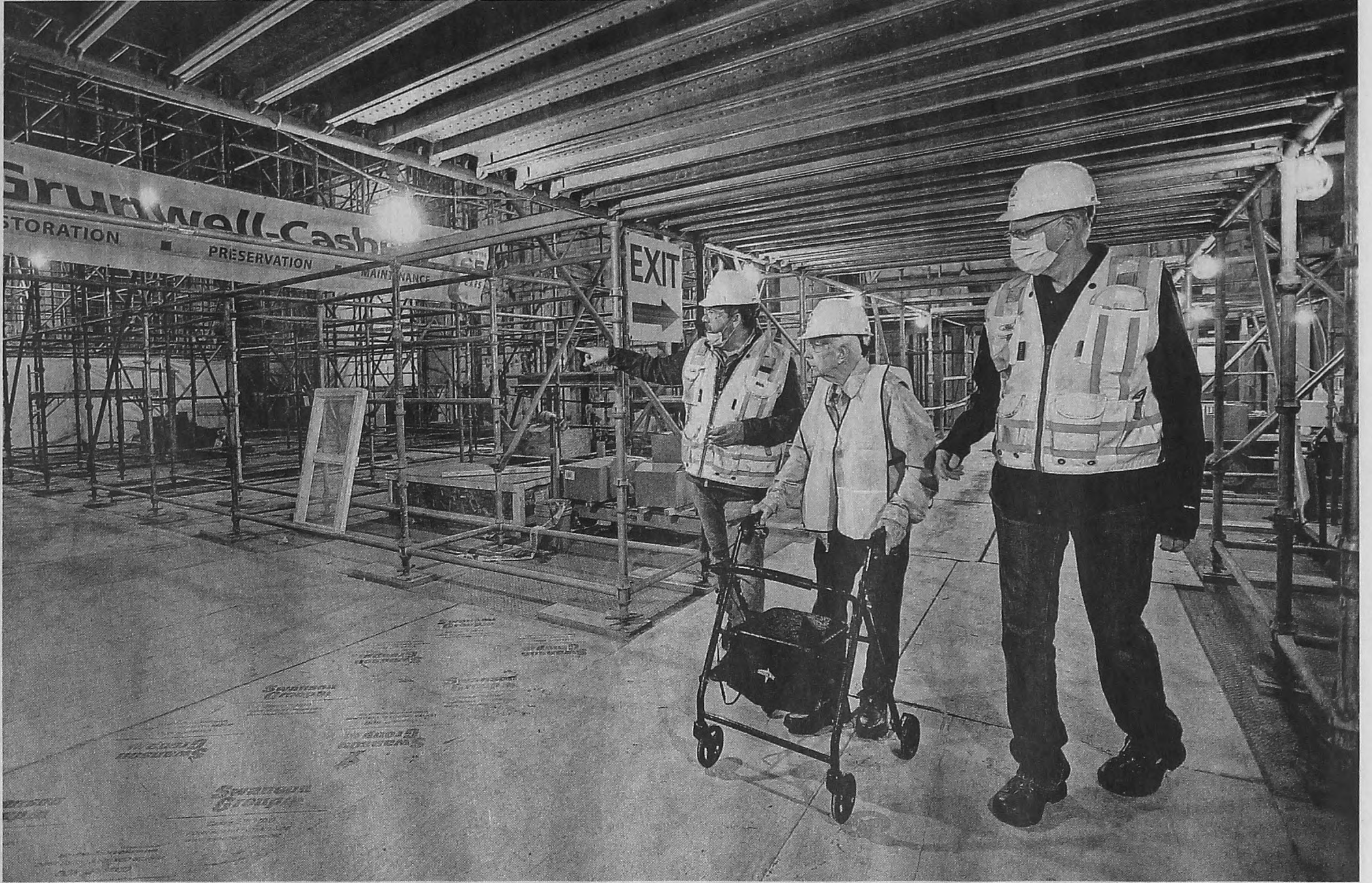
Michigan Central construction manager Richard Bardelli, left, and project manager Gary Marshall, right, guide Joe England for a tour inside of the Michigan Central Station in Detroit on Saturday. JUNFU HAN/DETROIT FREE PRESS
