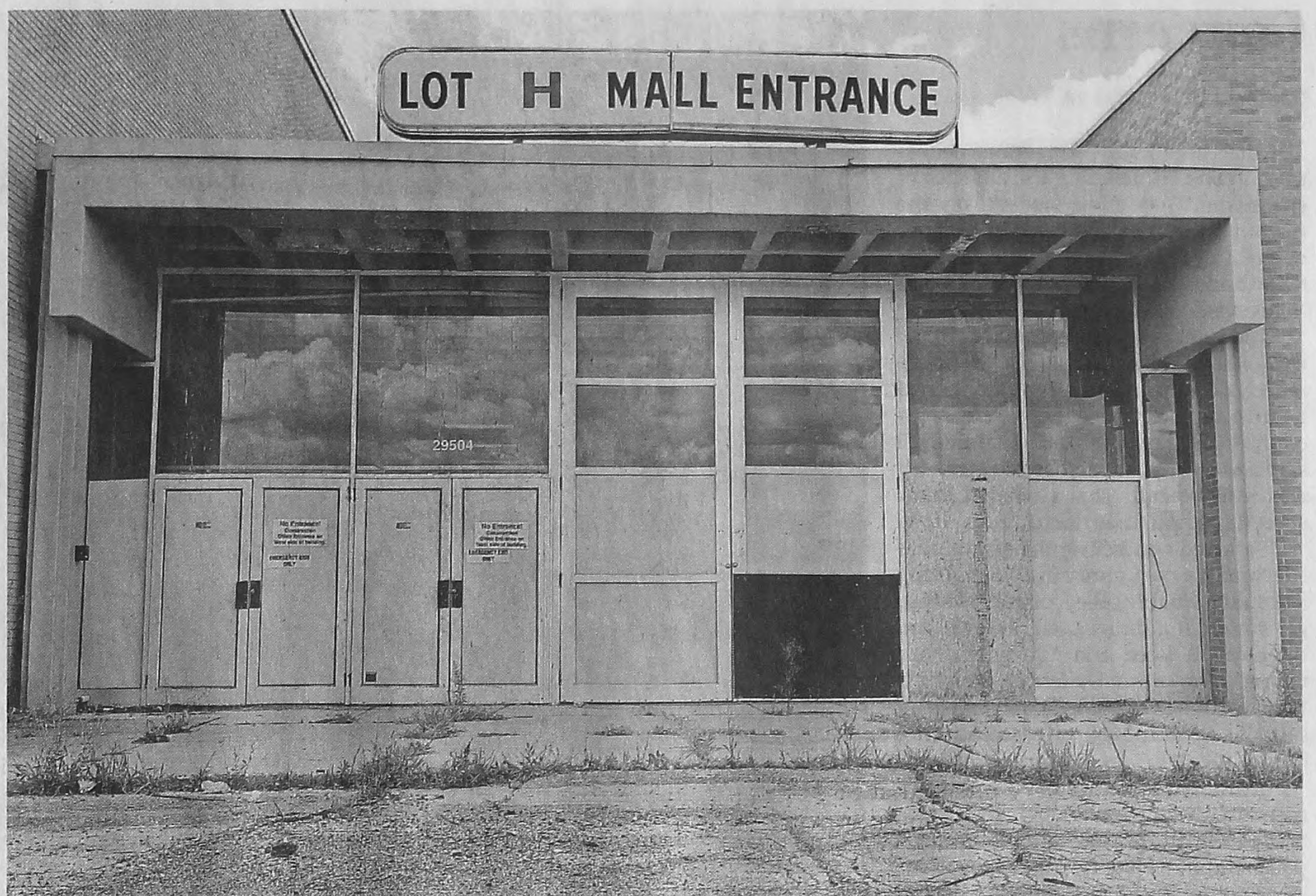
Sears was a big anchor store at the old Livonia Mall on Seven Mile Road, which later became Livonia Marketplace. Now this former entrance sits empty. PHOTOS BY ERIC SEALS/DETROIT FREE PRESS
