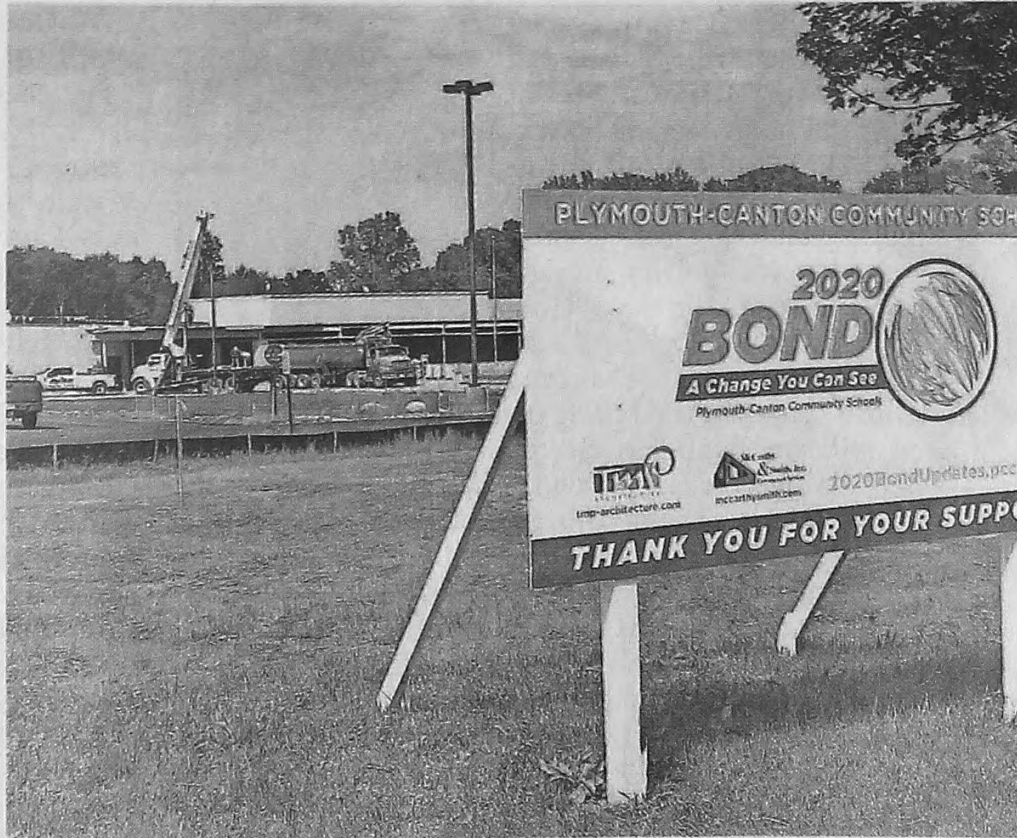
Paving on parking lot and student drop-off areas in front of Eriksson Elementary School is expected to be completed before the first day of school Sept. 7. ED WRIGHT/HOMETOWNLIFE.COM
