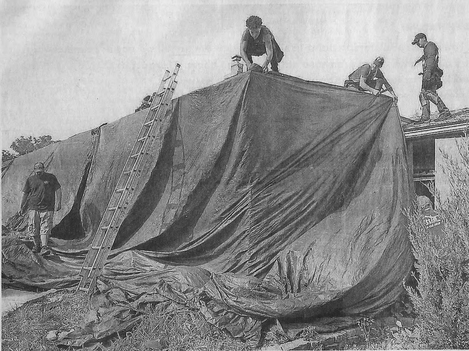
Tittle construction employees prepare to install a new roof at the Canton home of Army veteran Carson Middlebrook. ED WRIGHT/HOMETOWNLIFE.COM
