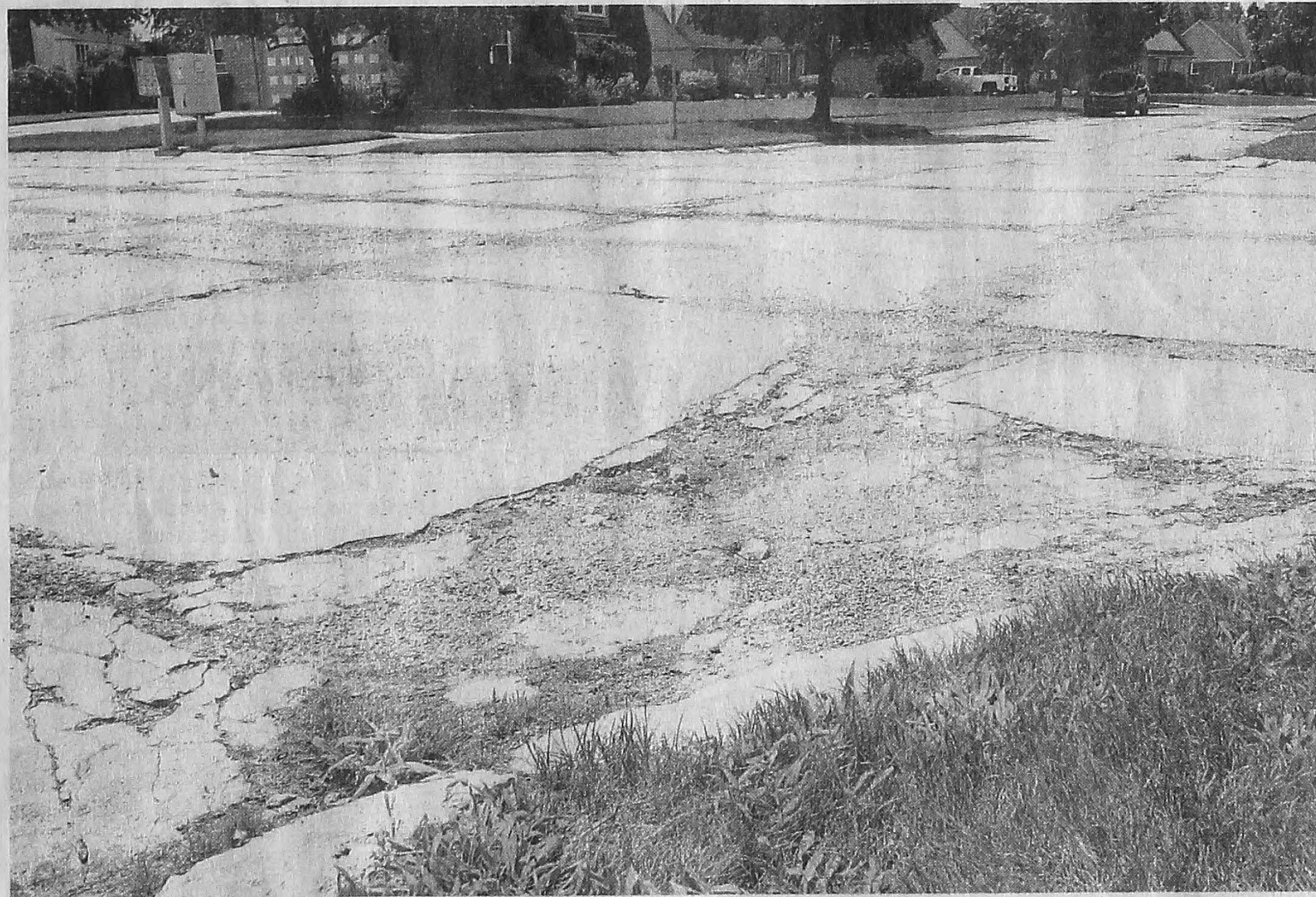
Homeowners along Oak Manor Court in Canton have dealt with a crumbling concrete road for years now and are hoping for a fix. This is the corner of Oak Manor and Swanmere. JOHN HEIDER/HOMETOWNLIFE.COM
