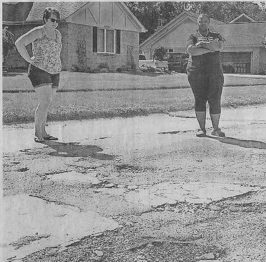
Canton residents Kortney Saxena (left) and Essence Uke stand along a deteriorating section of Swanmere Road in the Sunflower subdivision. ED WRIGHT | HOMETOWNLIFE.COM
