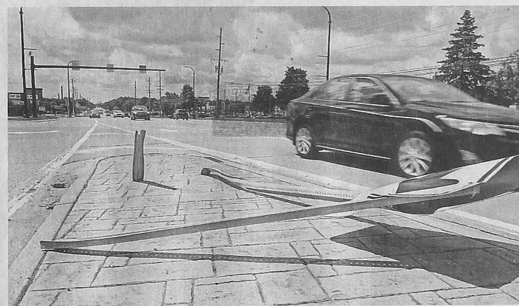
A crushed merge sign at Orchard Lake and 14 Mile attests to the intersection's danger caused by a lot of vehicles entering a very busy roundabout.
