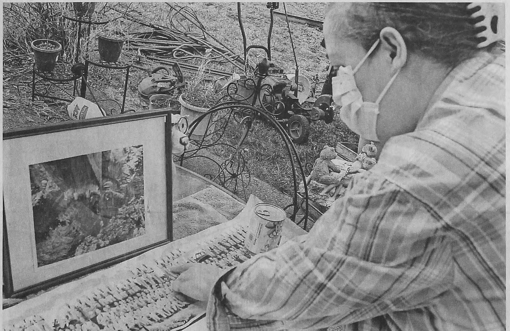
Kim Koester looks over photos of her late father, Robert Koester, from his time in the Army. She put the photos out to share with volunteers as they worked to demolish the garage at Robert's home in Livonia. DAVID VESELENAK/HOMETOWNLIFE.COM
