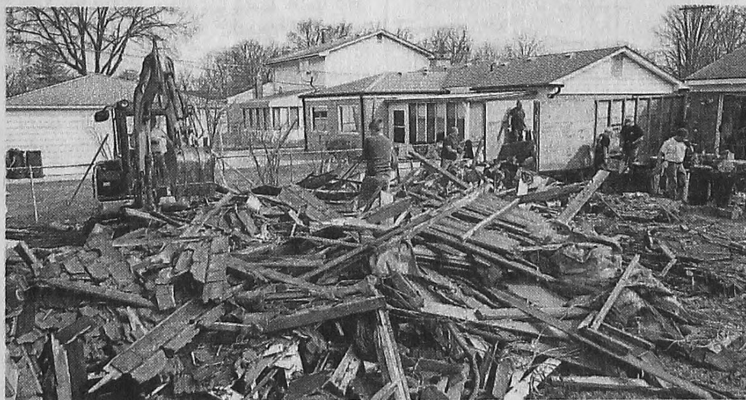
Volunteers work to sort the remains of the garage in Livonia on March 24.
