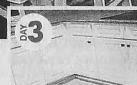
The installation is complete with the addition of new doors, molding and hardware
