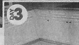
The installation is complete with the addition of new doors, molding and hardware
