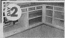
Your KURTIS craftsmen will cover all exposed surfaces with factory-finished materials.
