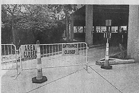
The lower level of Plymouth's two-decker parking lot west of Main Street is closed this week for repairs. JOHN HEIDER/HOMETOWNLIFE.COM
