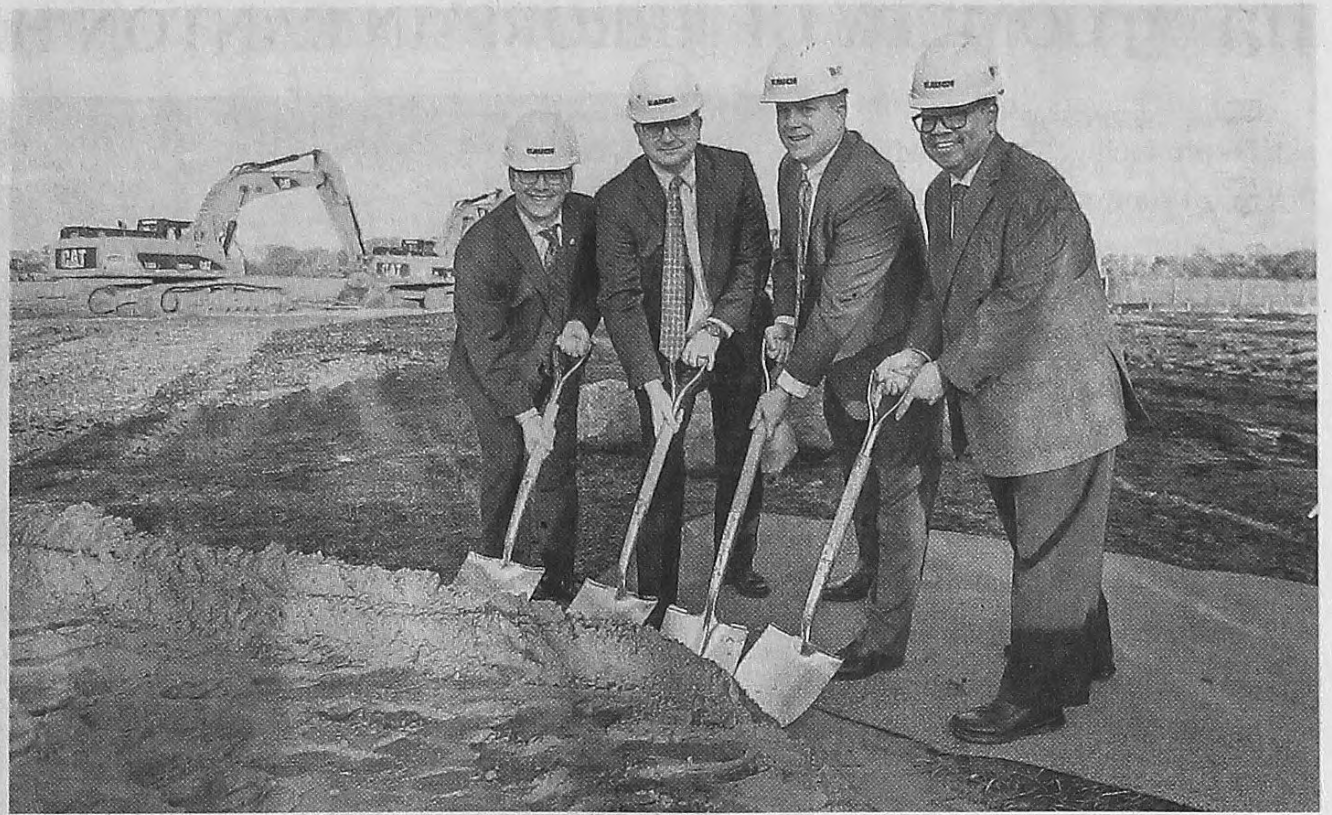
Leaders from Saint Joseph Mercy Health System, IHA and Schoolcraft College participate in a groundbreaking ceremony on the IHA & St. Joe's Livonia Medical Center on Nov. 18. From left are Rob Casalou, regional president and CEO, Trinity Health Michigan; Dr. Mark LePage, CEO, IHA; Brian Broderick, chair, Schoolcraft College Board of Trustees; and Dr. Conway A. Jeffress, president, Schoolcraft College. COURTESY OF ST. JOSEPH MERCY HEALTH SYSTEM
