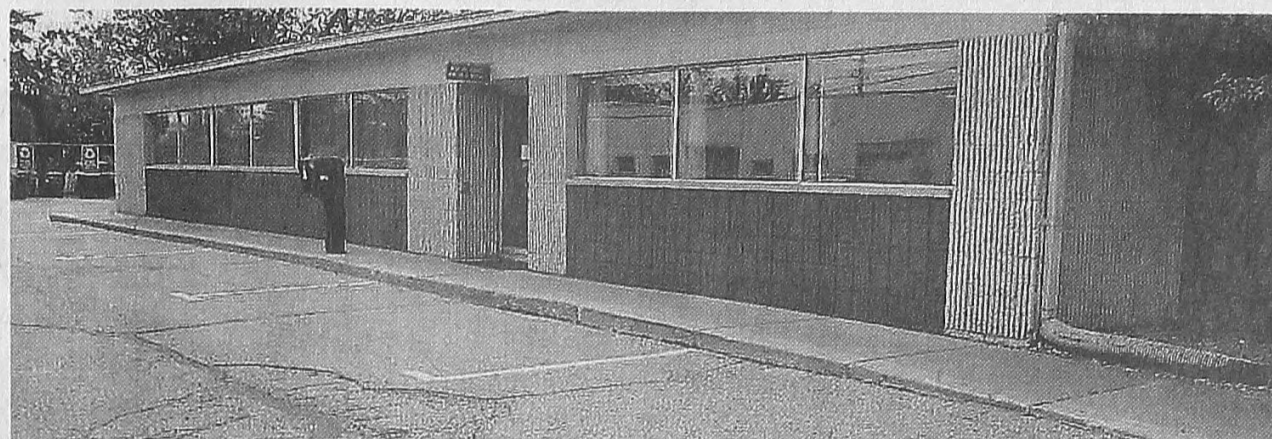
This photo of the Plymouth municipal offices shows the problematic area before a rain garden was installed. MATTHEW BERTRAND
