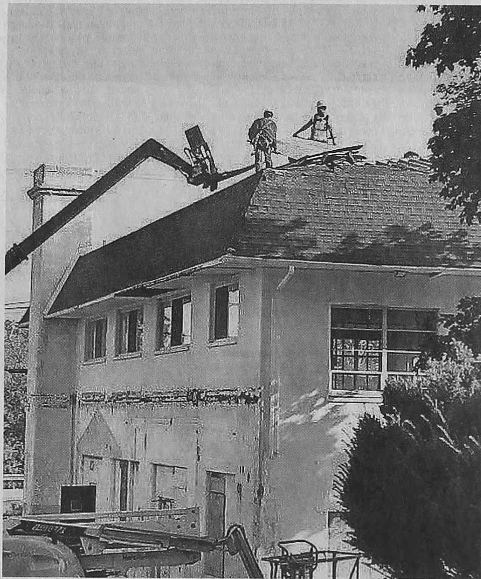
Crews work on the roof of the arts factory on the old Ford property in Cherry Hill Village.
