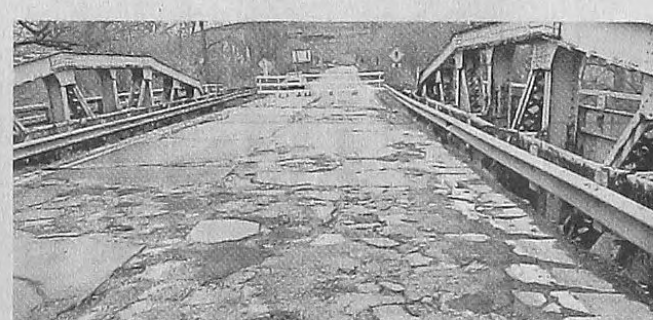
CANTON TOWNSHIP An engineering firm has recommended this Lilley Road bridge in Canton be replaced.
