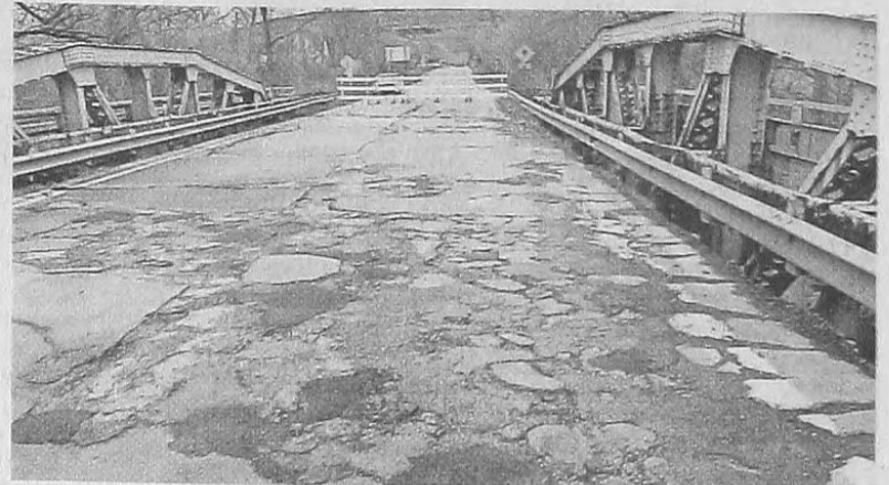
CANTON DEPARTMENT OF PUBLIC WORKS Wayne County has closed this bridge on Lilley, north of Michigan Avenue, to determine whether it is safe.
