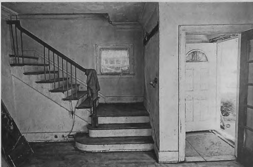
The entrance to the home, with stairs leading to the second floor.
