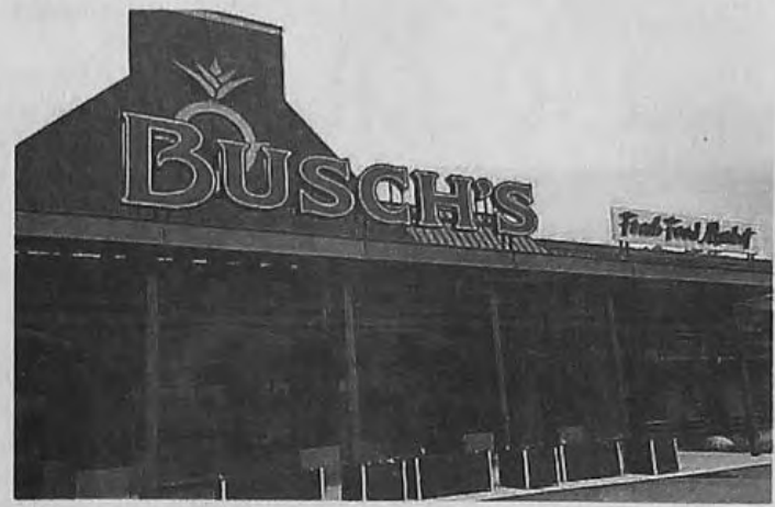
DARRELL CLEM Interior demolition is occurring on the Busch's Fresh Food Market site in Canton.
