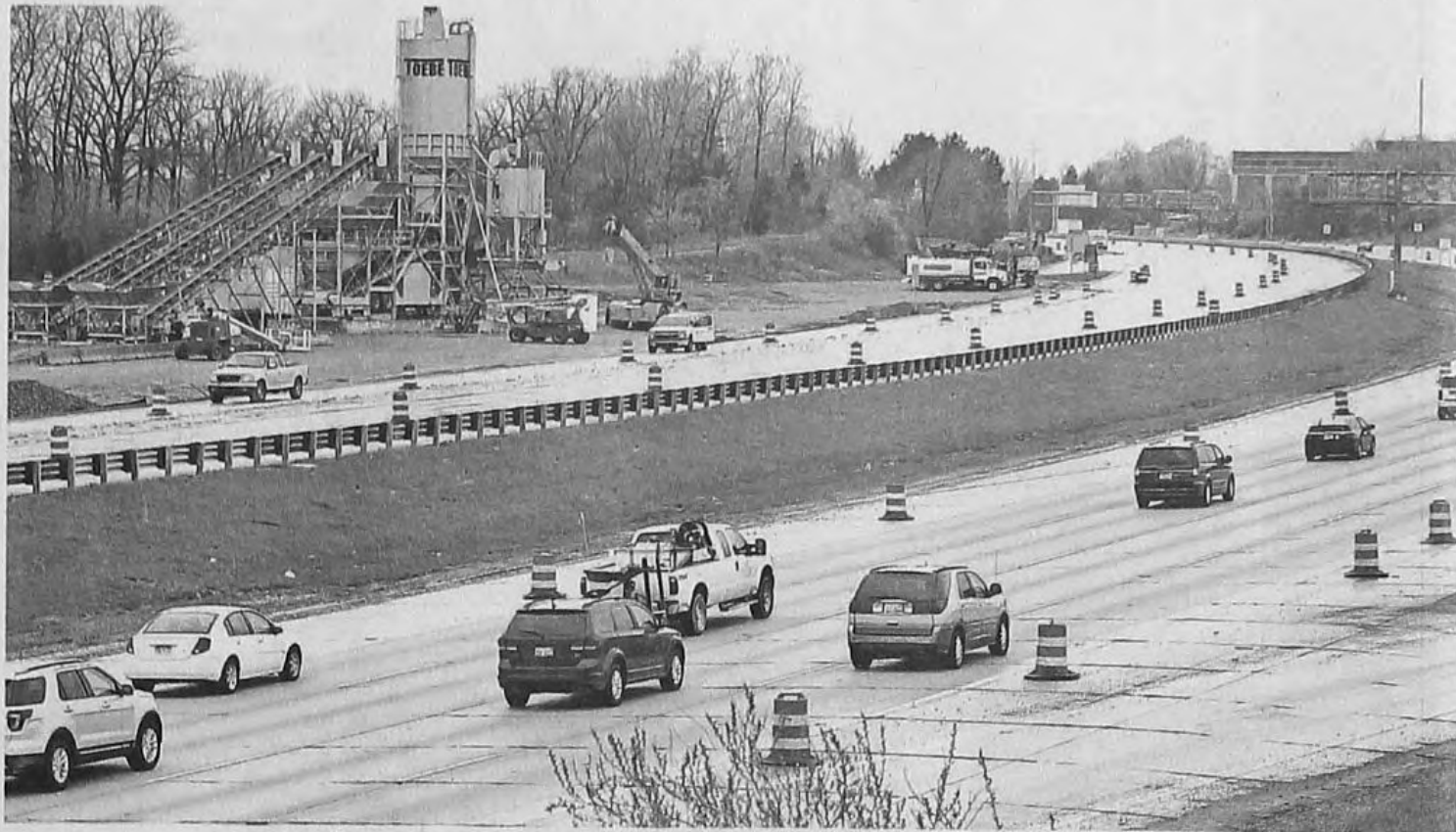
Northbound traffic was normal at mid-morning Monday. There was no southbound traffic other than construction-related vehicles. The concrete plant is up and ready.
