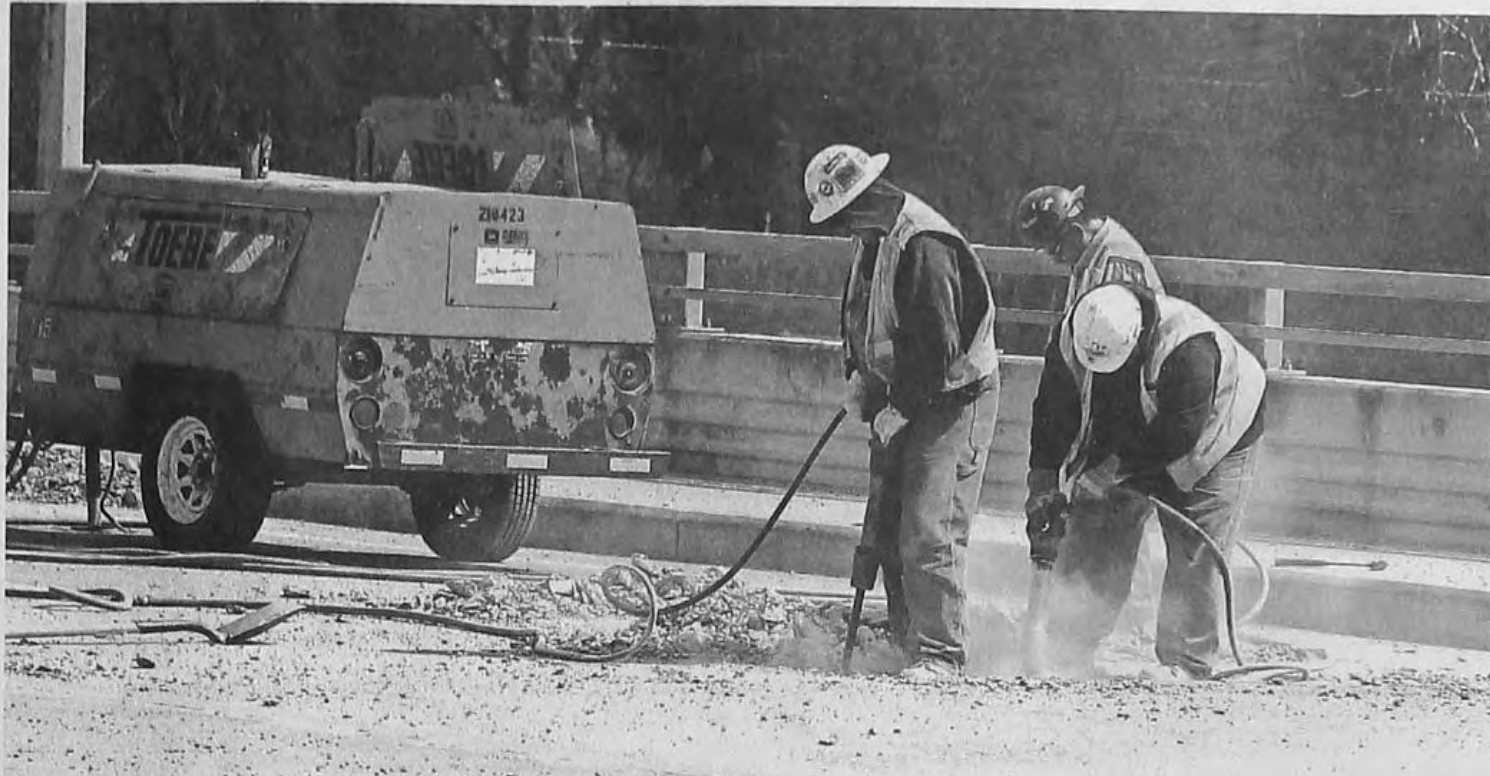
The eastbound ramp over I-275 at Seven Mile is already closed as workers begin removing and replacing its road surface. The effort is part of the reconstruction efforts on the major highway that lies between Northville, Novi and Livonia and Farmington Hills.
