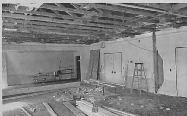
After the Griffin family bought the Northrop-Sassaman Funeral Home, they "took it down to the studs" to renovate it.
