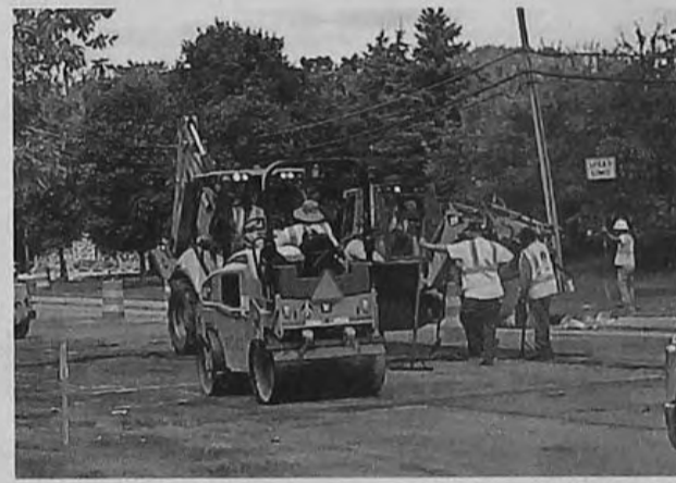
Work crews have started repairing Lilley Road between Warren and Joy in Canton.
