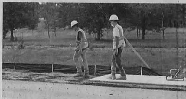
BILL BRESLER | STAFF PHOTOGRAPHER Construction workers are continuing their efforts on Ford Road in Canton.
