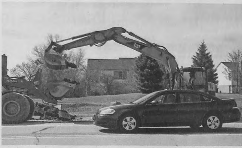
Cars travel through the Cherry Hill Road construction zone. The project runs from Canton Center Road west to Beck Road.
