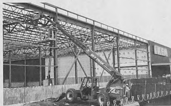
BILL BRESLER | STAFF PHOTOGRAPHER Work is progressing on IKEA Canton's 44,000-square-foot expansion.
