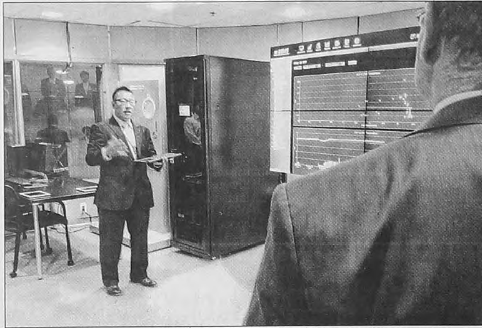
Project manager Trey Lim from Smart and Green Controls in Plymouth discusses the K-MEG project at its unveiling.
