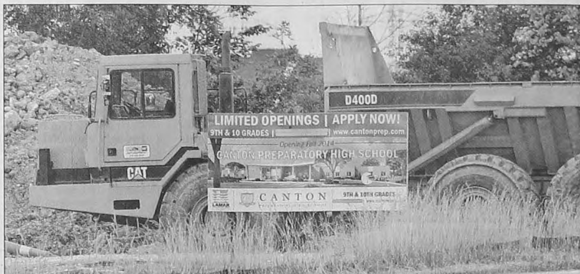
Officials say construction on Canton Preparatory High School, the charter school being built on Cherry Hill in Canton, won't be affected by the fact its general contractor, Lamar Construction Co., filed this week for bankruptcy. PHOTOS BY BILL BRESLER | STAFF PHOTOGRAPHER
