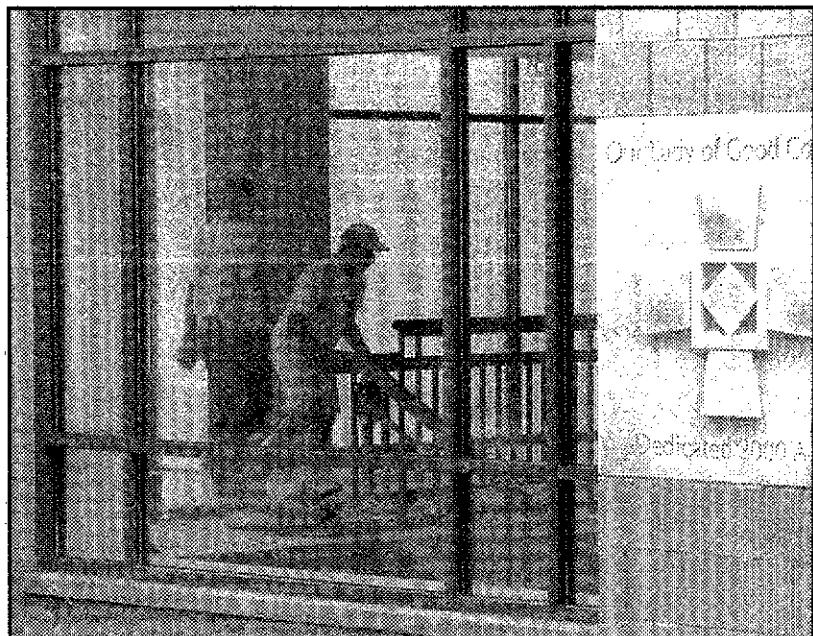
Finishing touches: Construction workers paint the railings inside the new building. The cornerstone, at right, holds a time capsule for the future.
