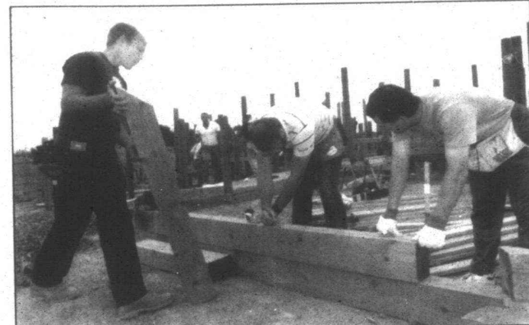
Measuring: Steve Henke (center) and Justin Klumper (right) measure timber while constructing Heritage Hideout, Canton's playscape. Helping out is Dave Forsman (left).
