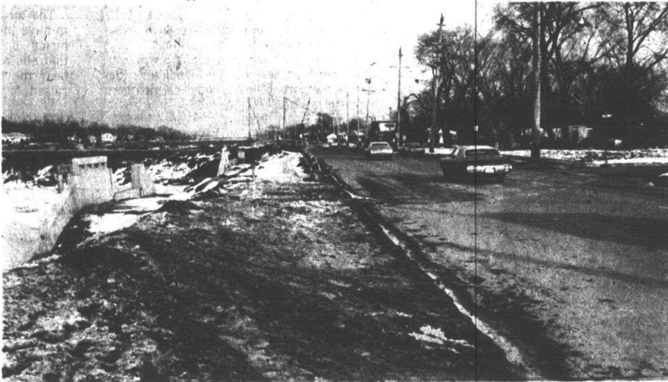
THE LACK OF protective barriers along Schoolcraft road between Norborne and Centralia allowed another vehicle to land in the deep ditch being dug for the freeway. This accident, involving a car driven by Ray Sher-
